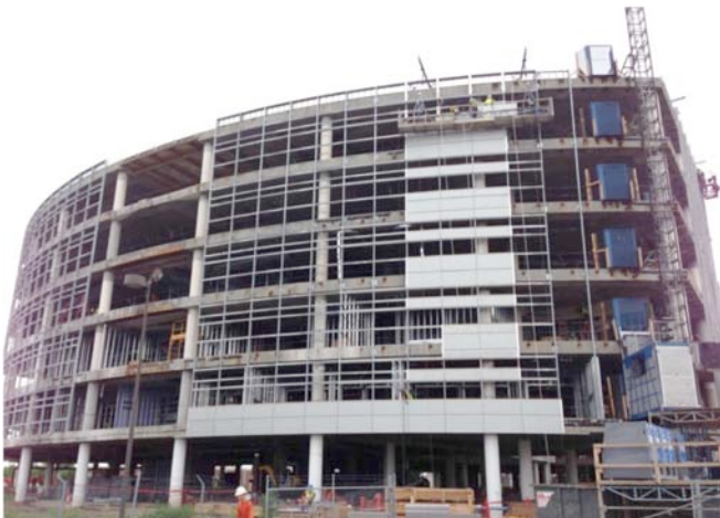
Photograph 1: Insulated Metal Panel System I —Concrete frame infilled with metal framing and clad with insulated metal panels.
