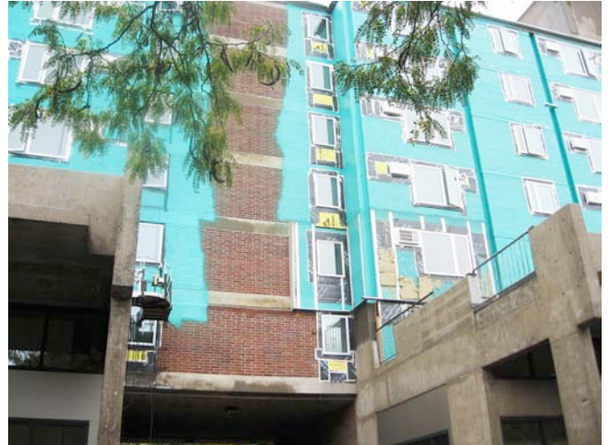
Photograph 6: Retrofit Metal Panel —With retrofit approaches it is common to apply a fluid water and air control layer directly to the masonry. Note the sheet membrane transition between the field of the wall and the replacement glazing system.
