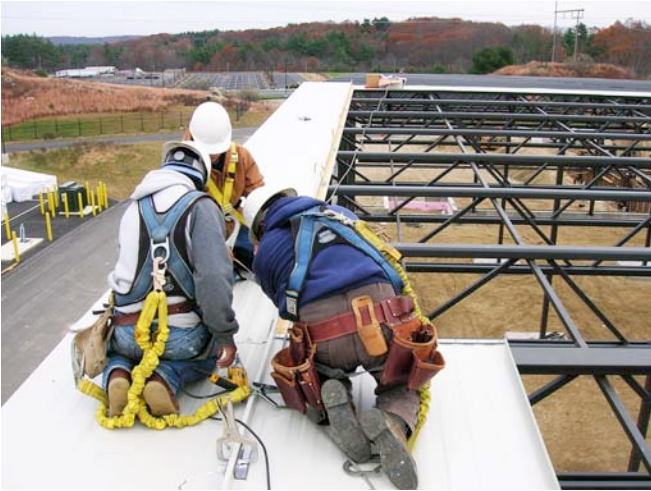
Photograph 4: Insulated Metal Roof Panel —Installation of roof panels “crimping” the “standing seams”.
