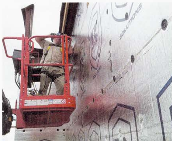
Exterior CI comes in many forms: polyiso, expandable polystyrene, extruded polystyrene, along with spray foam are some of the choices. Each available non-faced or with multiple options for facers such as aluminum foil or fiberglass laminated to the surface. Image courtesy of Rodenhouse Inc.
