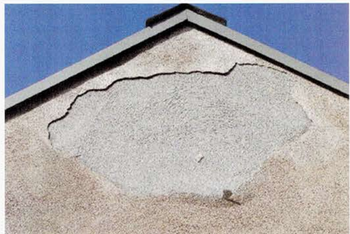
Stucco failure discovered on Schooner Cove condominiums in South Tampa, Fla., built by DR Horton. Courtesy of KIS Consulting, LLC.
